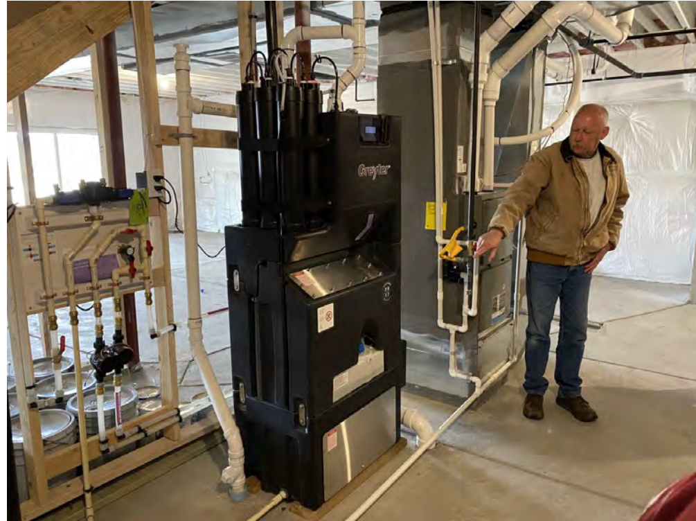
First Gray Water Systems hit Castle Rock in 2021/2022
