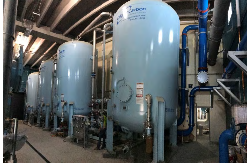
Granular Activated Carbon Filters at Plum Creek Water Purification Facility
