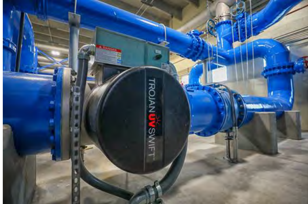
Ultraviolet Radiation at Plum Creek Water Purification Facility
